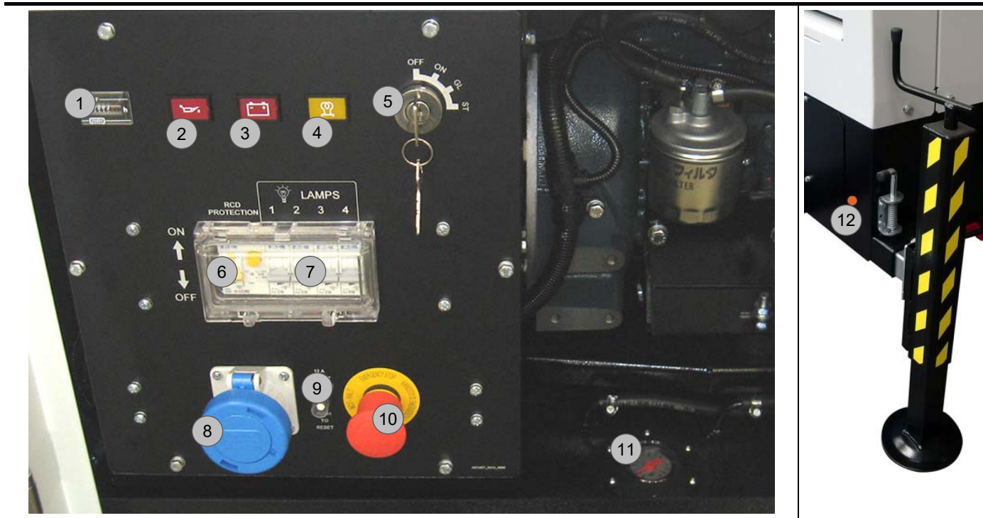
Control panel__Panel de control
